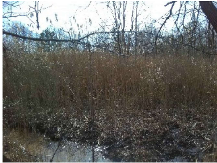
A EXISTING OVERGROWN AND FILLED DETENTION BASIN.
