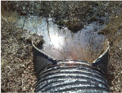
B EXISTING OUTLET PIPE (NO OUTLET STRUCTURE)
